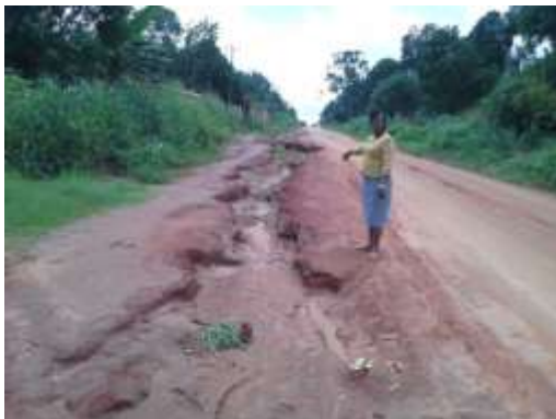
Splash Erosion (First Stage of erosion) along Ideato North and South Express way
